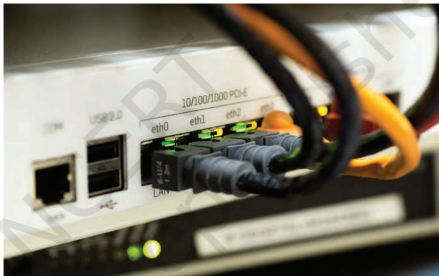
Figure 5.9: Cables connected to a network switch
